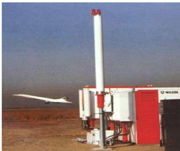
Station DME au sol
